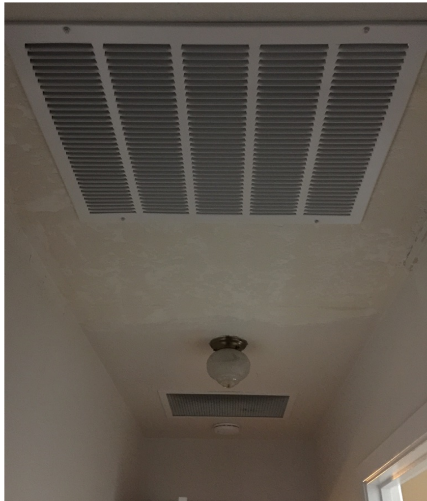
Cold Air Return (close) Whole House Fan (far)
