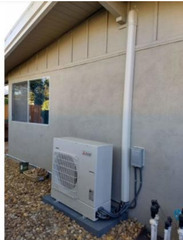
Air Source Heat Pump Mini Split (ductless)
