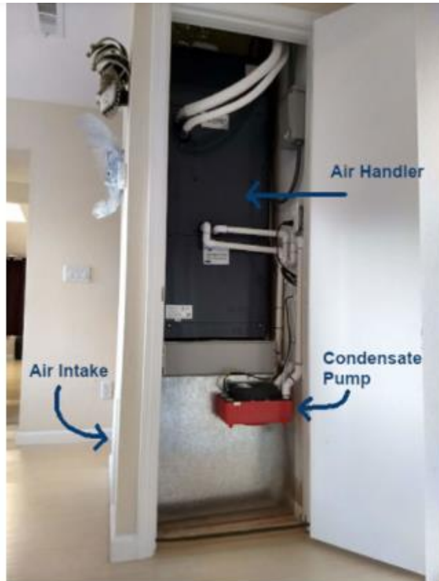
Central Air Source Heat Pump (uses air ducts)
